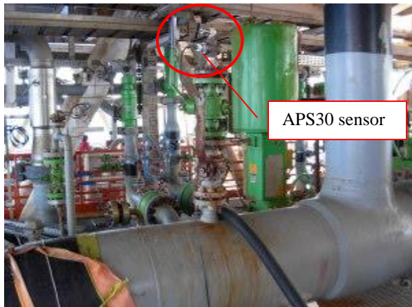
Fig. 27: APS30 mounted on the arrival of the riser on the platform
