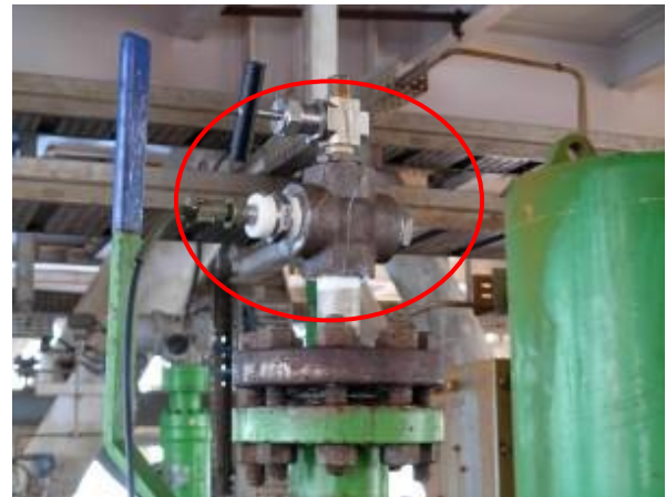
Fig. 28: APS30 sensor with its drilling valve
